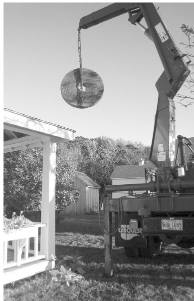
The Gamage grindstone is carefully lowered into place at SBHS with the help of Plummer Excavation.
